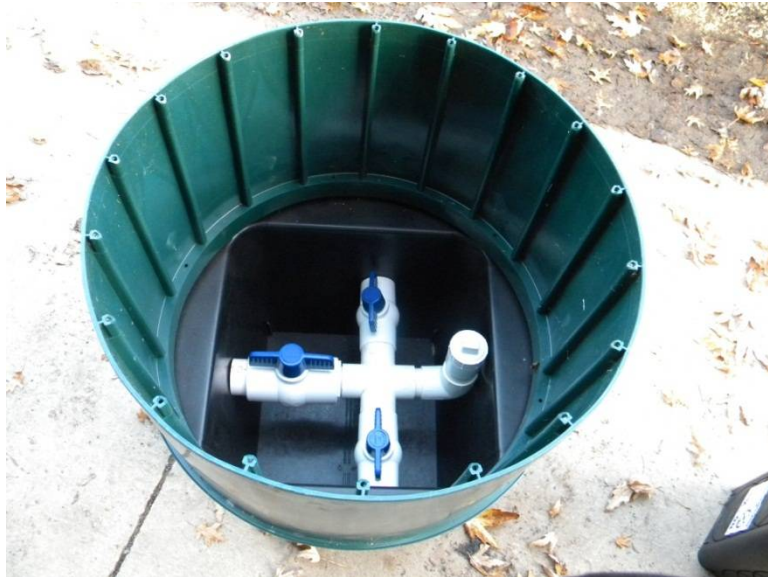
Figure 7. Service box within the manifold line
