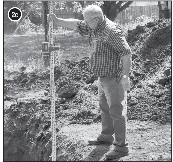
Make sure the excavation is stable, smooth, level, and free from debris, rocks, and sharp objects.
