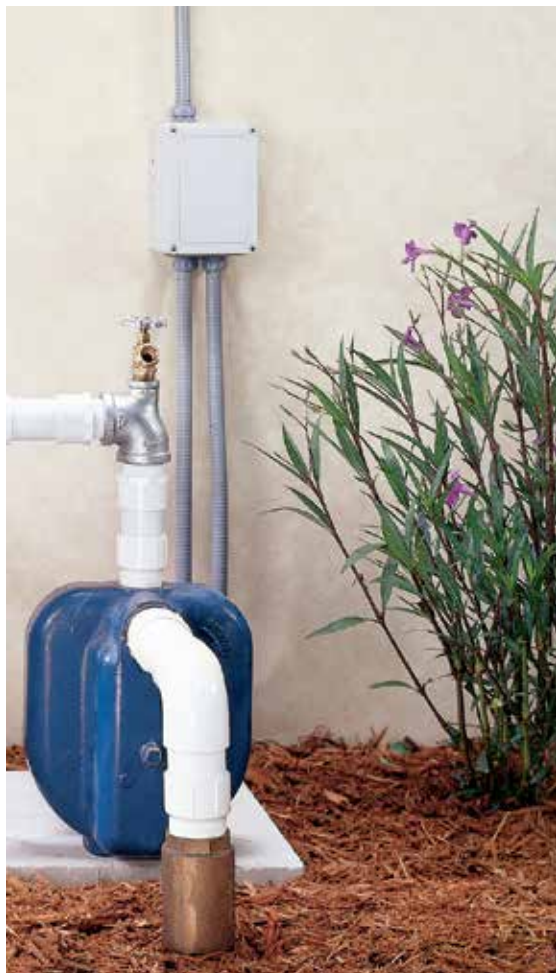
pump start relays
